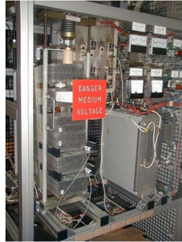
Fig. A-3. A medium voltage test rack in the University of Wisconsin lab.
